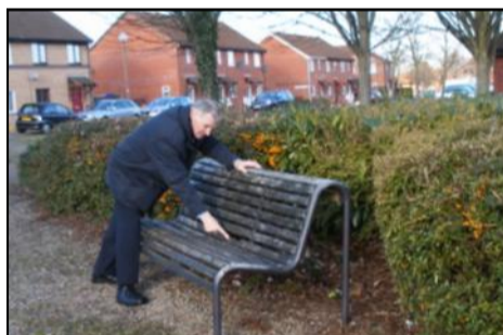
Pictured left Cllr Alan Richards highlights a broken timber in this public bench in Giffard Park.
