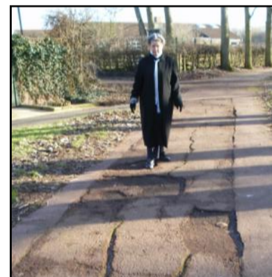
Cllr Christine Zealley stands by a hazardous section of red way in Great Linford. Cllr Zealley said "These badly surfaced redways are probably deterring residents from their using bikes?"
